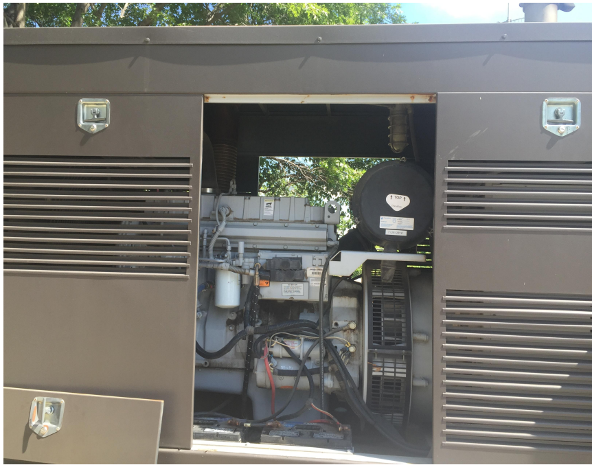
Standby Power Generator
