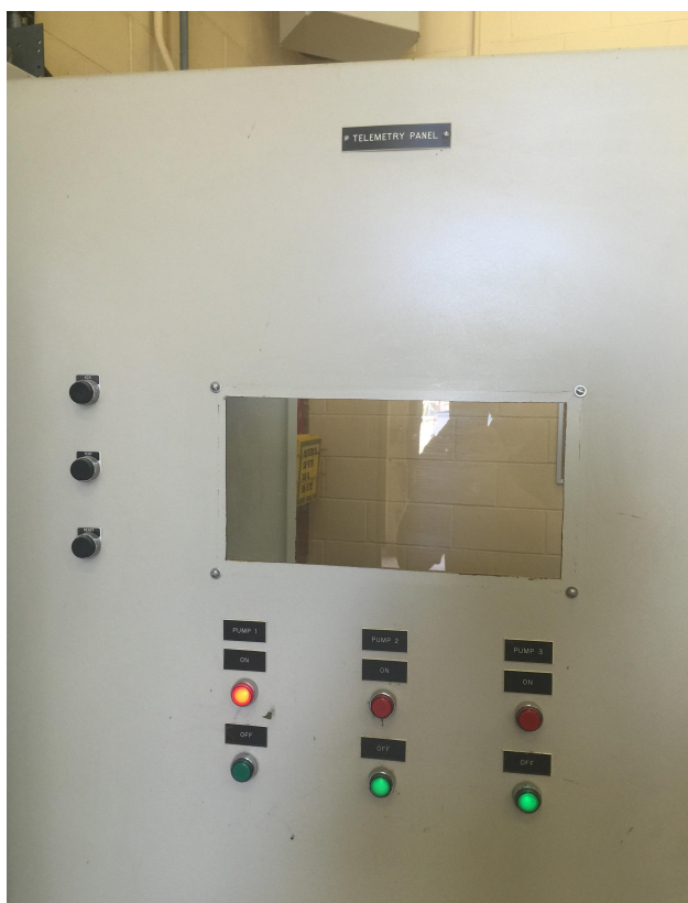
Telemetry Panel - Exterior Door Panel
