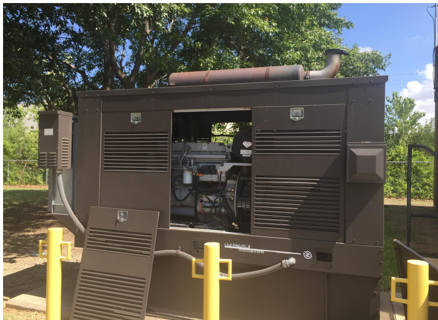
Standby Power Generator
