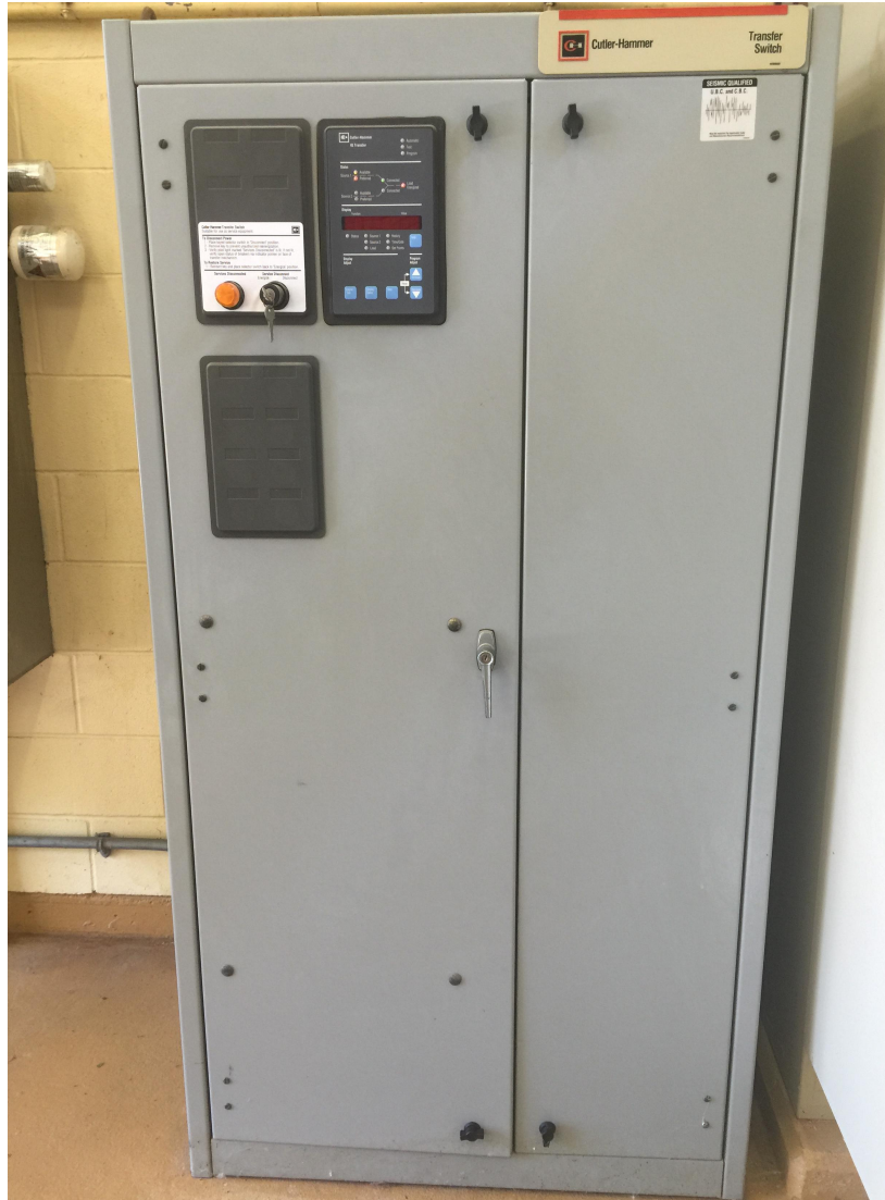
Automatic Transfer Switch
