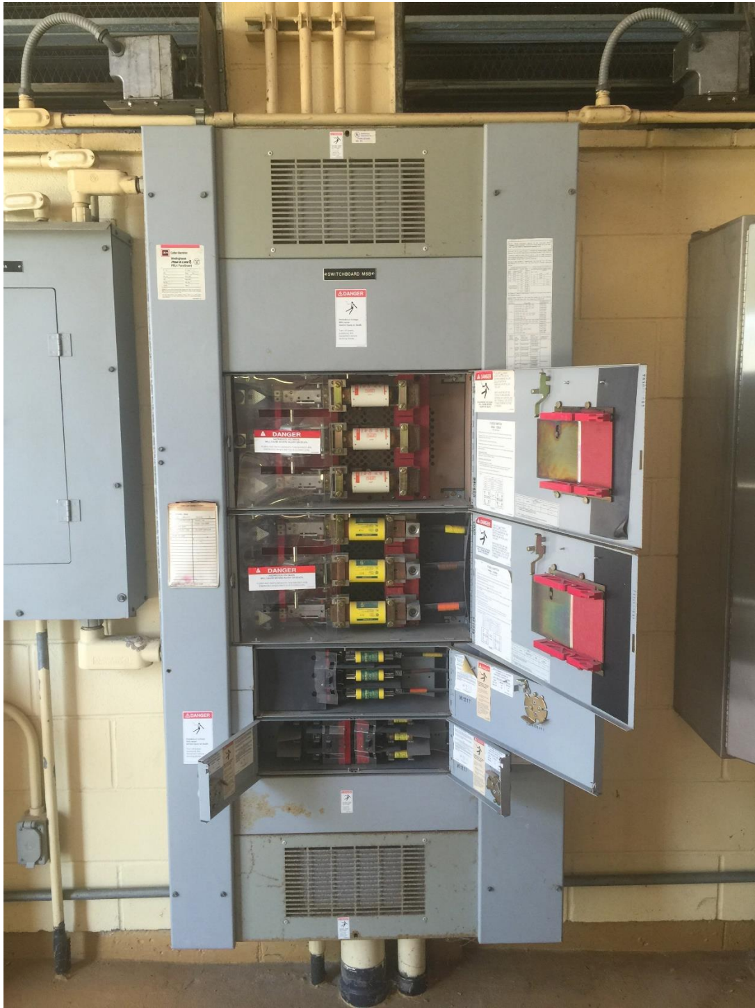
Figure 1-3: Existing Switchboard MSB
