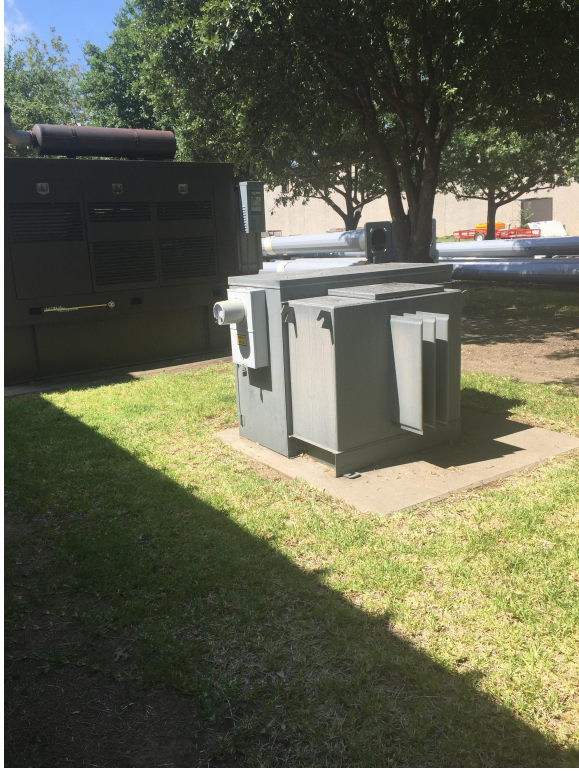
Service Transformer and Meter
