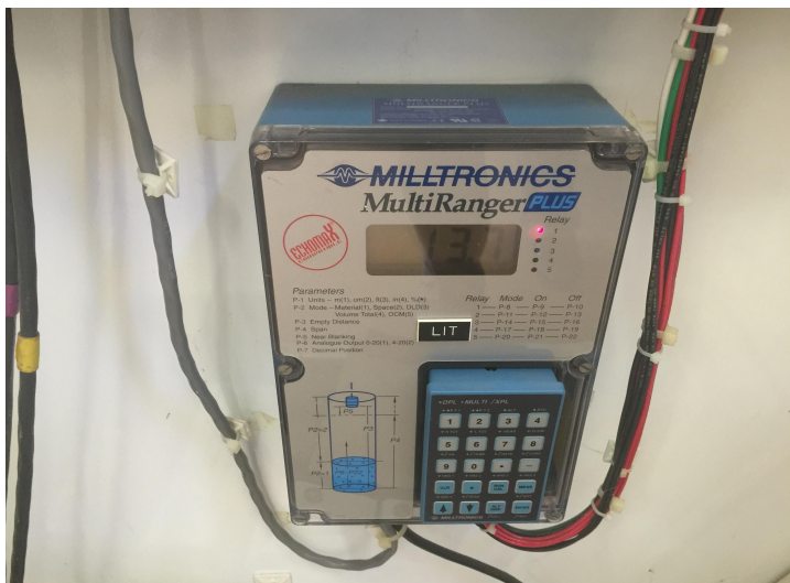
Telemetry Panel Level Transmitter
