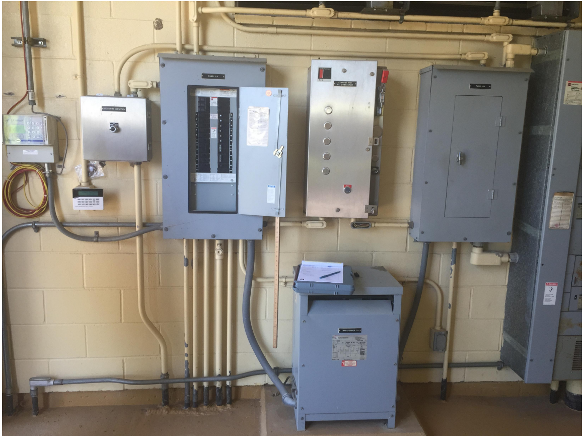
Dry Type Transformer, Panel HA, Panel LA and Exhaust Fan Panel
