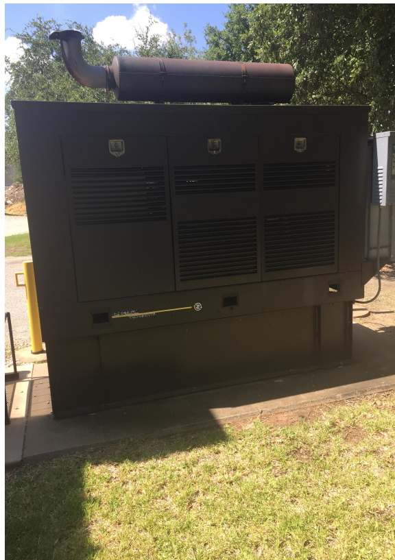
Standby Power Generator
