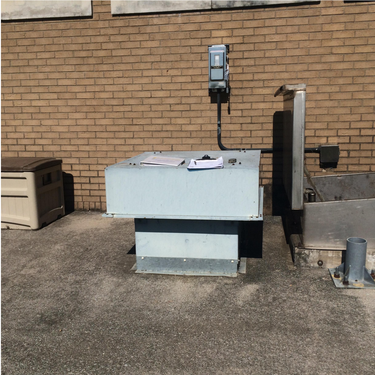
Wet Well Exhaust Fan (F-3)
