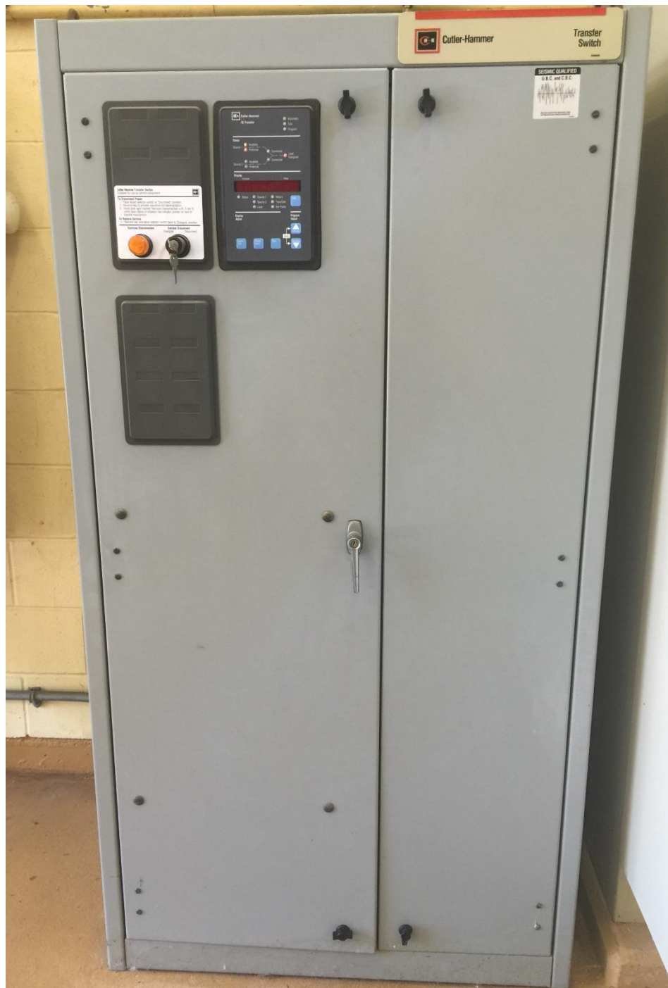
Figure 1-4: Existing Automatic Transfer Switch
