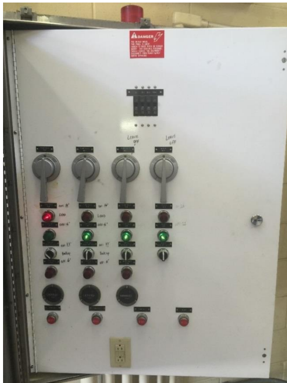
Figure 2-1: Pump Control Panel
