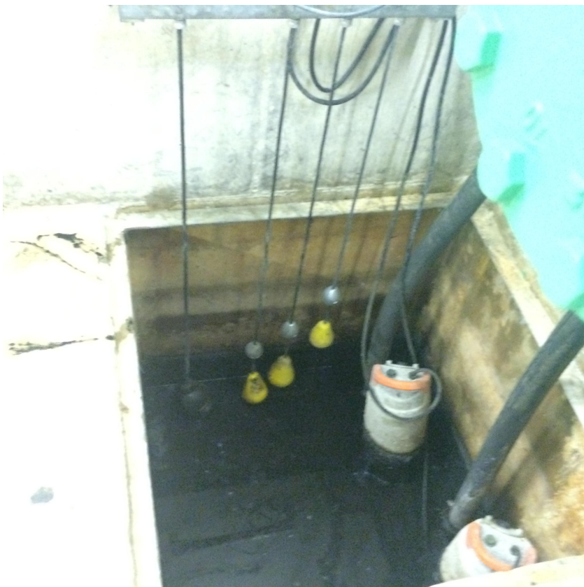
Sump Pumps 1 and 2
