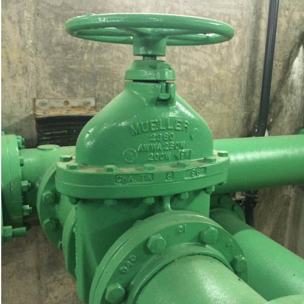
Pump 1 Discharge Isolation Gate Valve (8")
