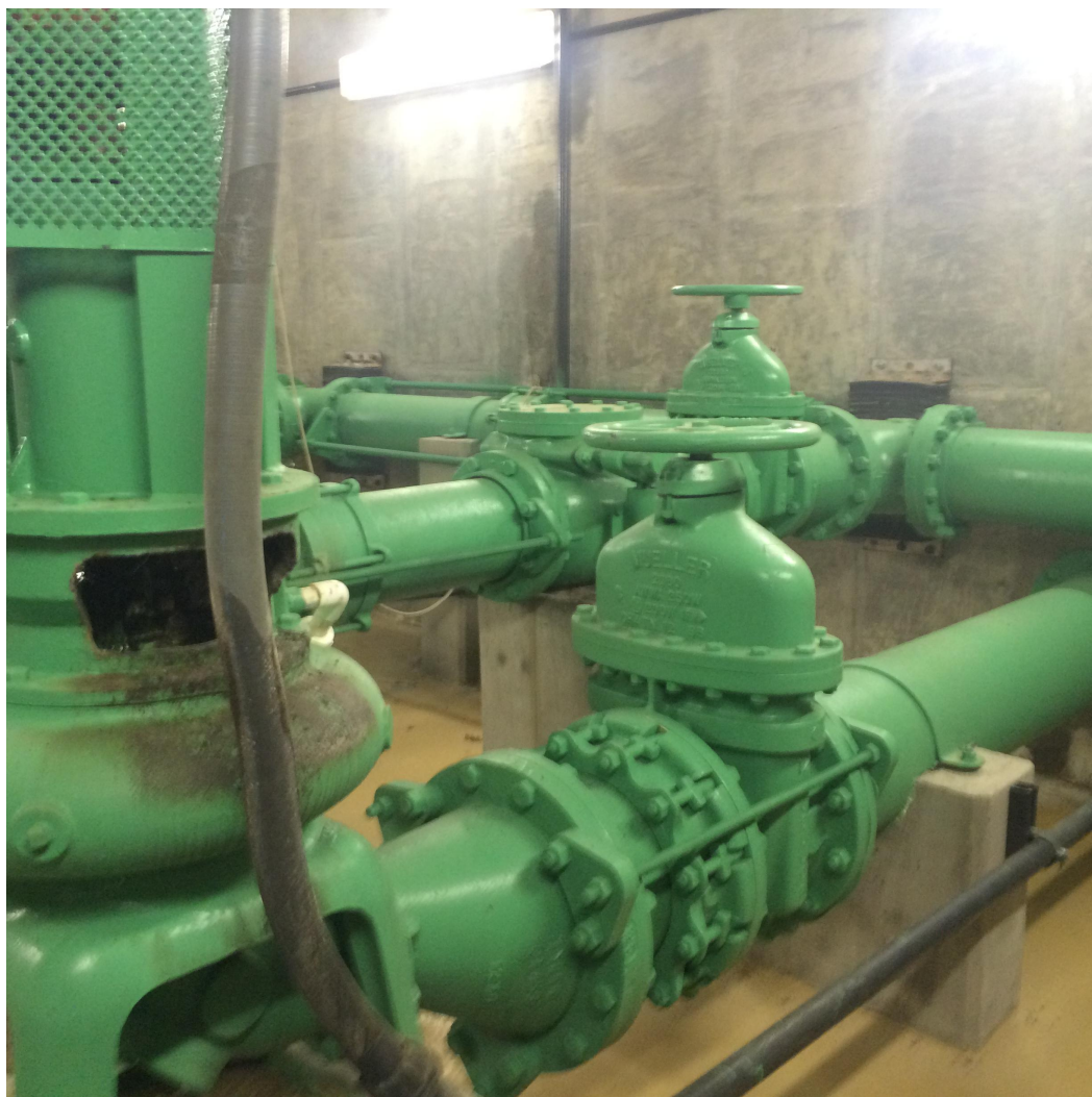
Pump 2 Suction Isolation Gate Valve (12")
