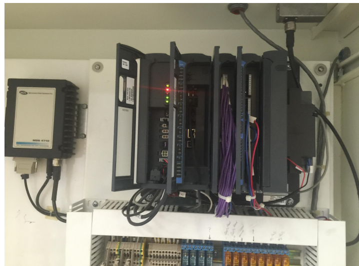
Telemetry Panel Motorola PLC and MDS Radio
