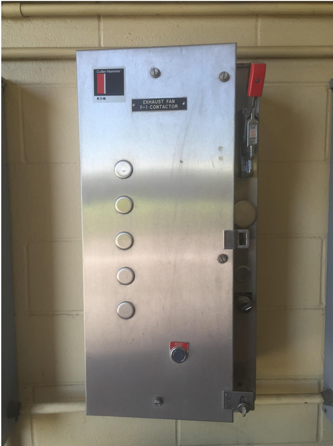
Figure 1-2: Existing MSB-3 (Exhaust Fan Control Panel)
