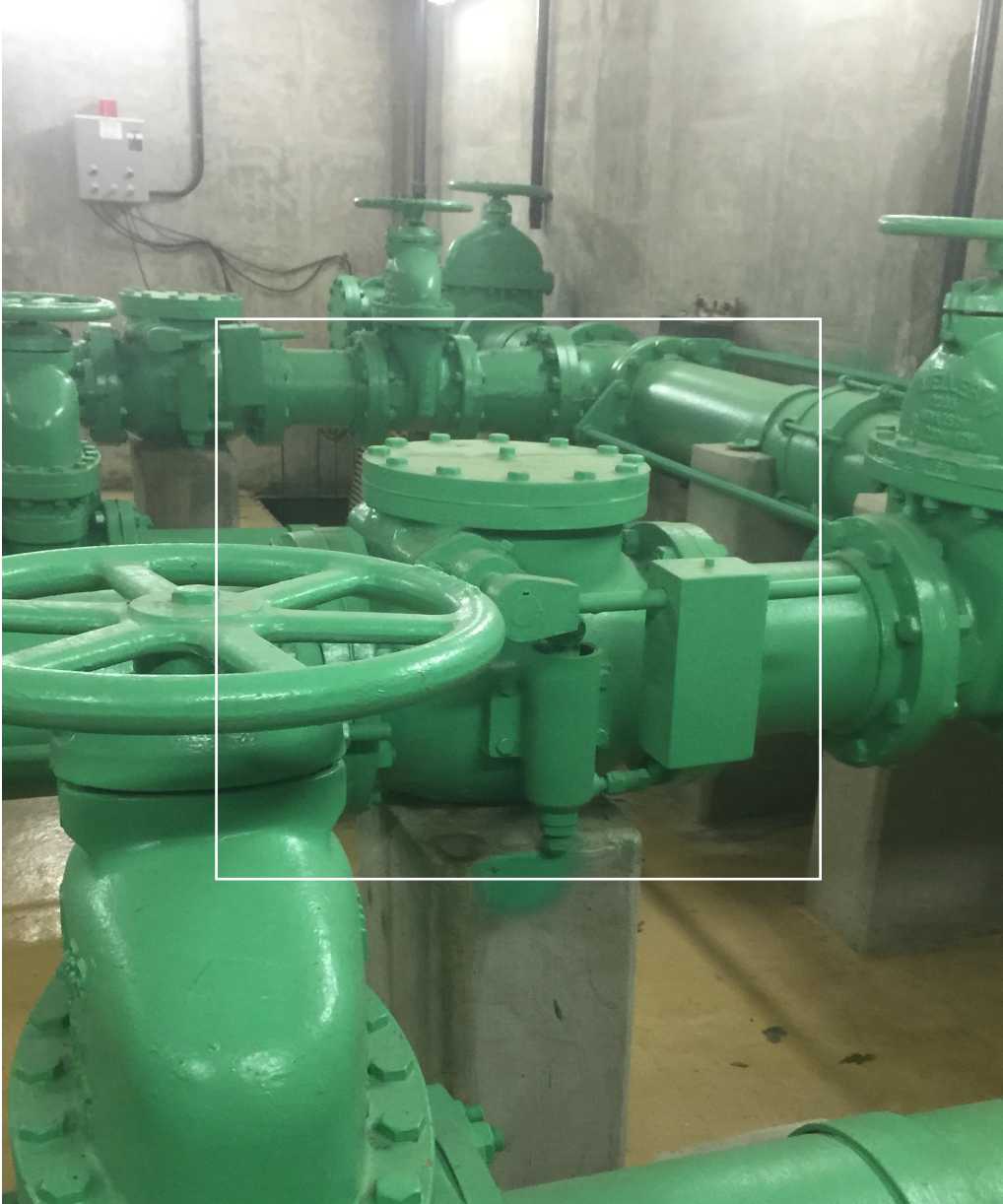
Pump 1 Discharge Check Valve (8")
