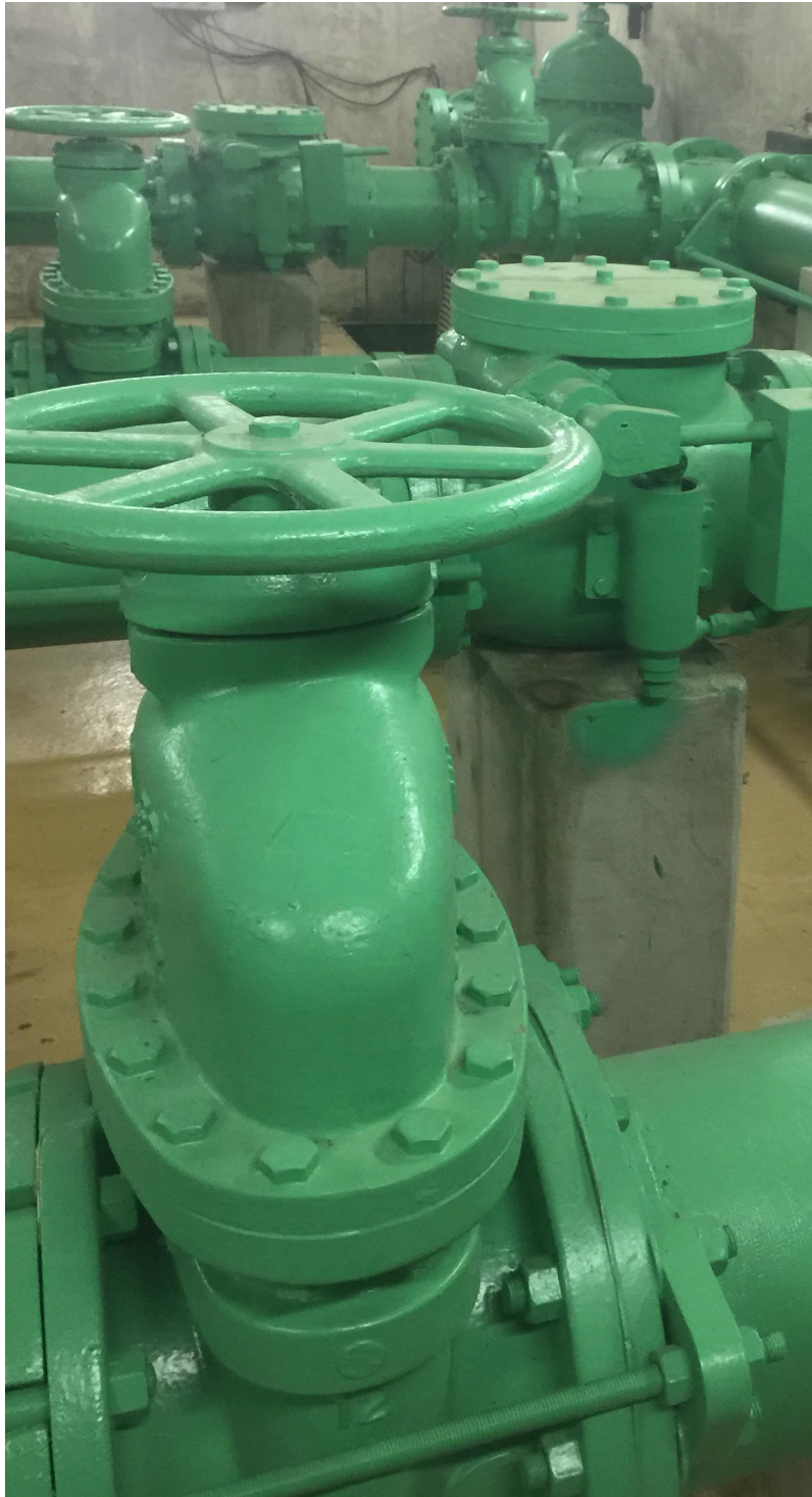
Pump 1 Suction Isolation Gate Valve (12")
