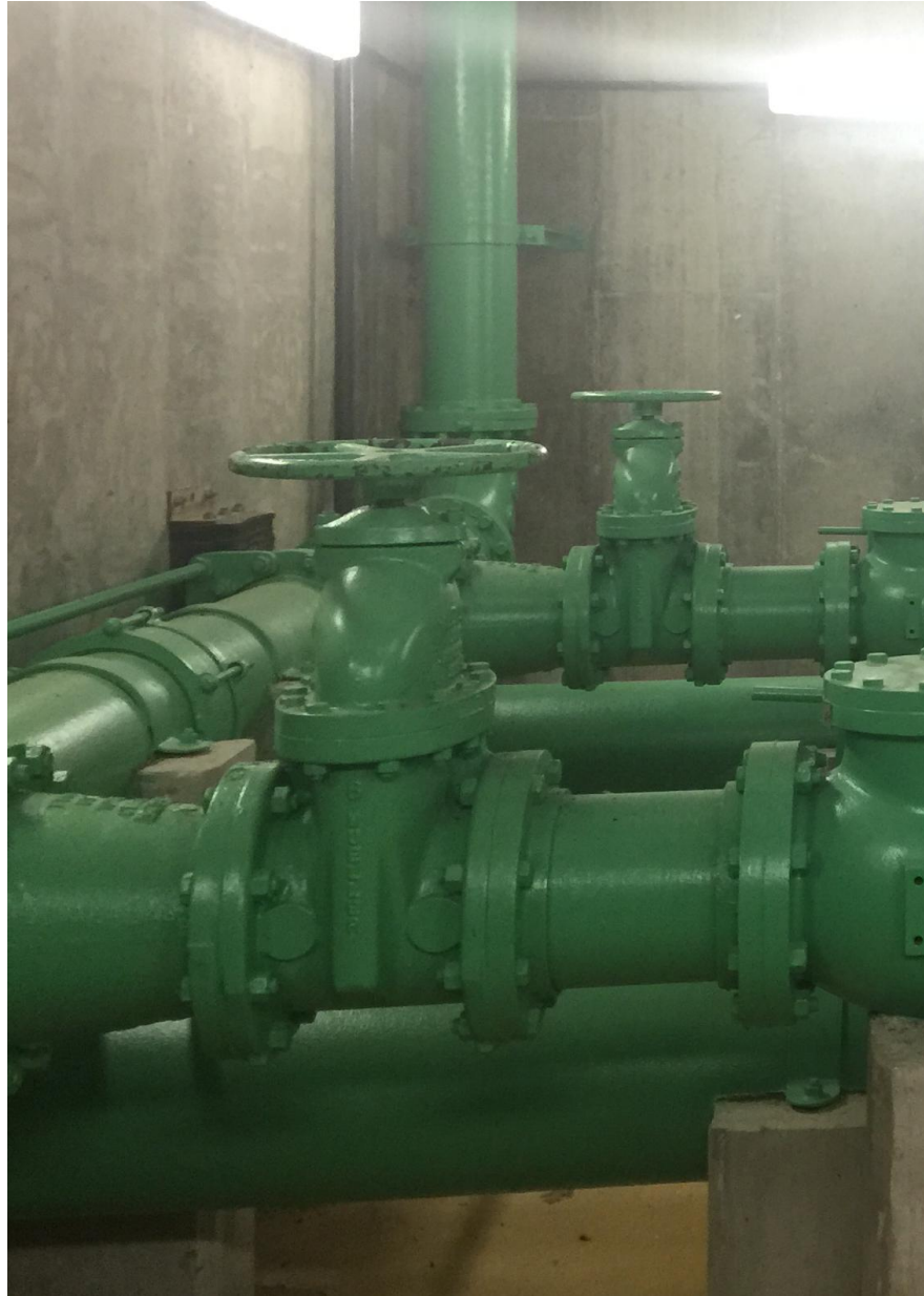
Pump 2 Discharge Isolation Gate Valve (8")
