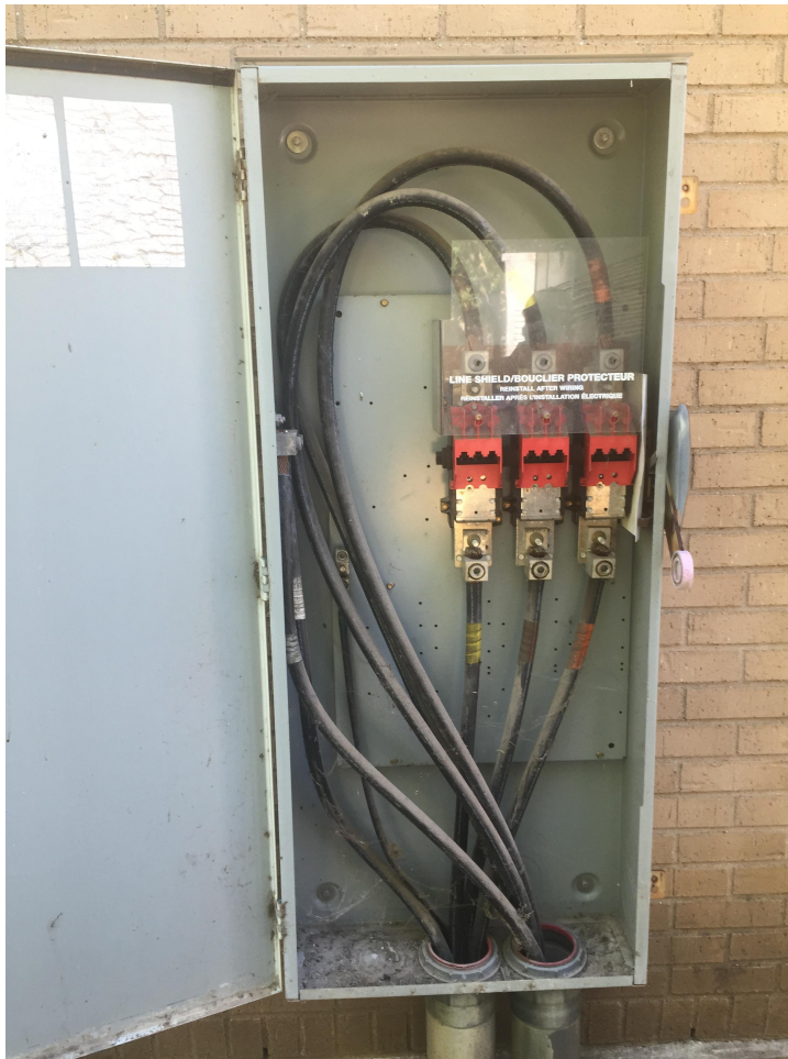
Emergency Generator Disconnect
