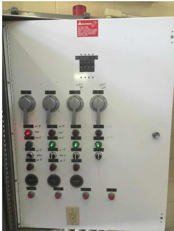
Panel MCCA - Interior Swingout Door with Controls
