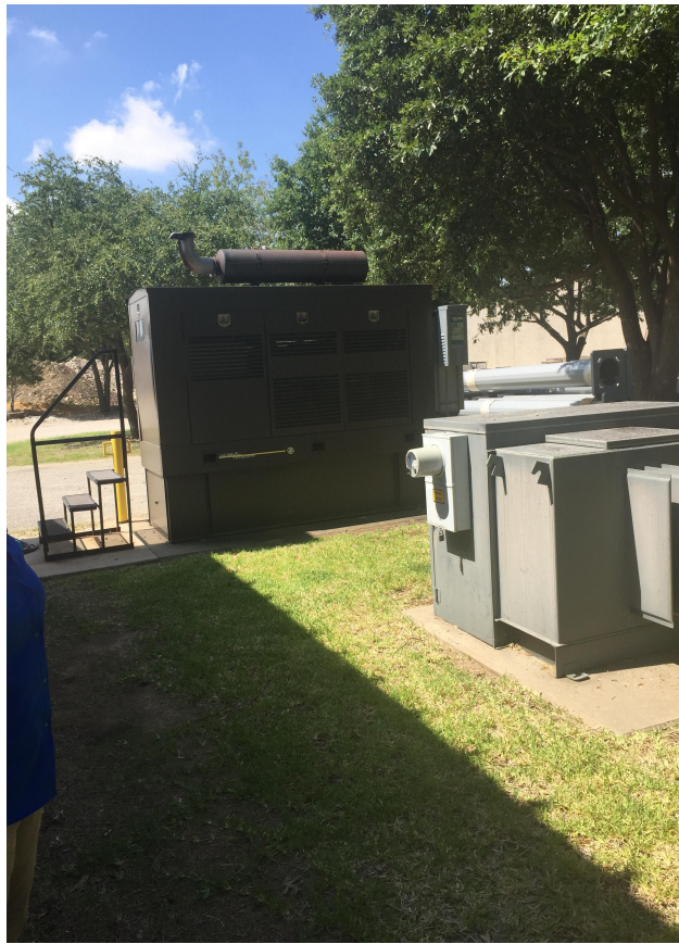
Standby Power Generator and Transformer
