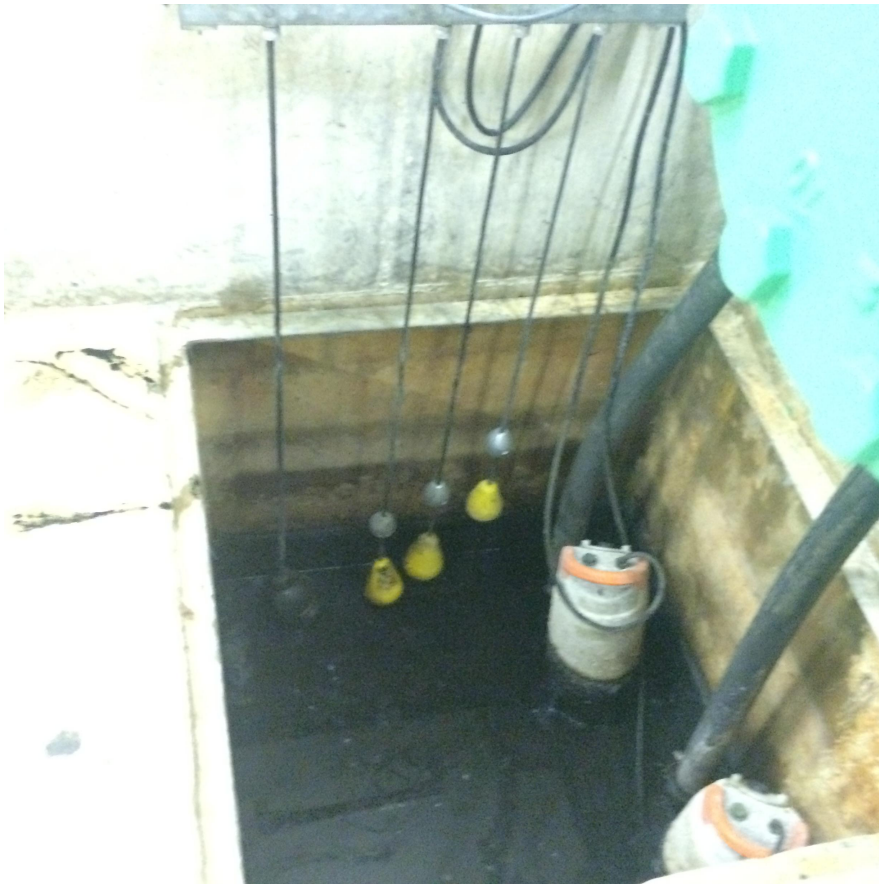
Sump Pumps 1 and 2
