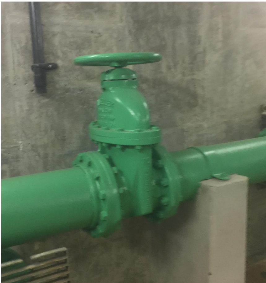
Discharge Header Gate Valve (10")
