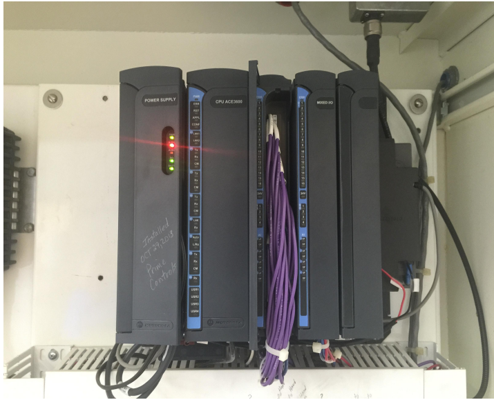
Telemetry Panel Motorola PLC
